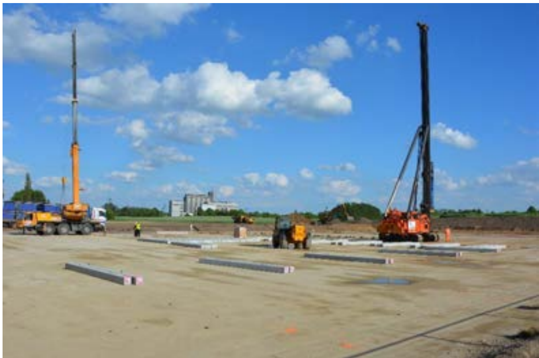
Fig A6. Example of a cement bound platform (level smooth surface – beware of ponding)
