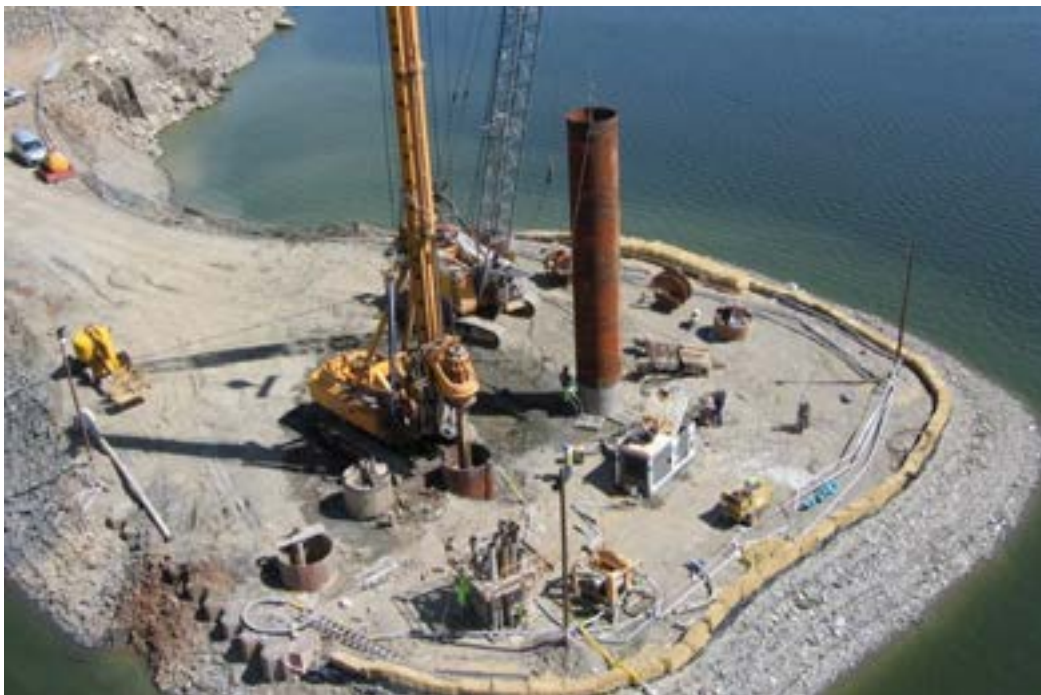
Fig A8. Example of edge protection around the platform to protect the environment
