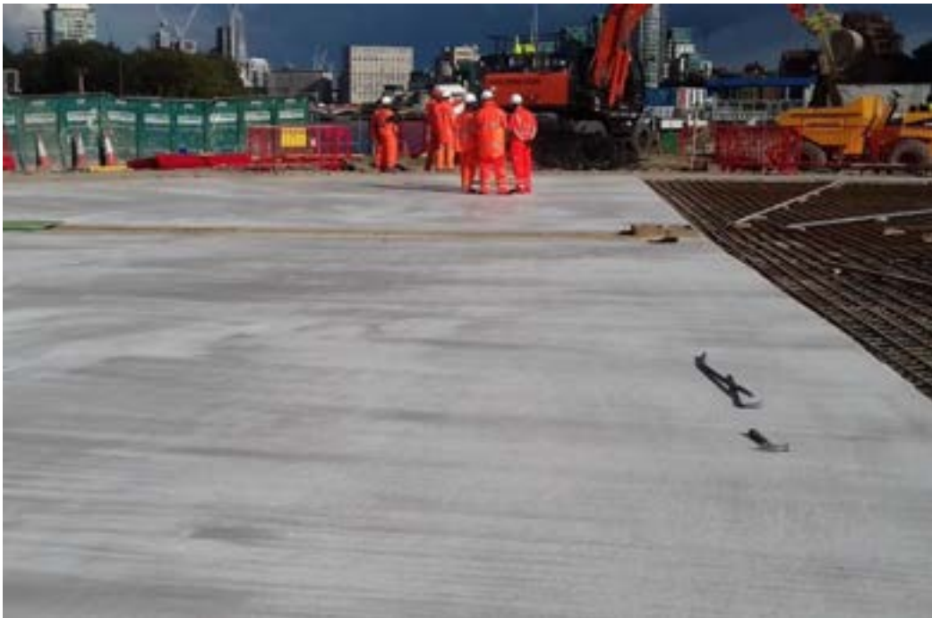
Fig A7. Example of a reinforced concrete platform (with drainage in centre)
