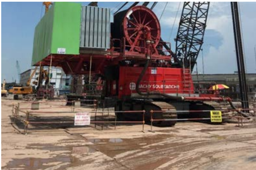
Fig A4. Platform overlaid by steel plates (beware of creating a slippery surface)
